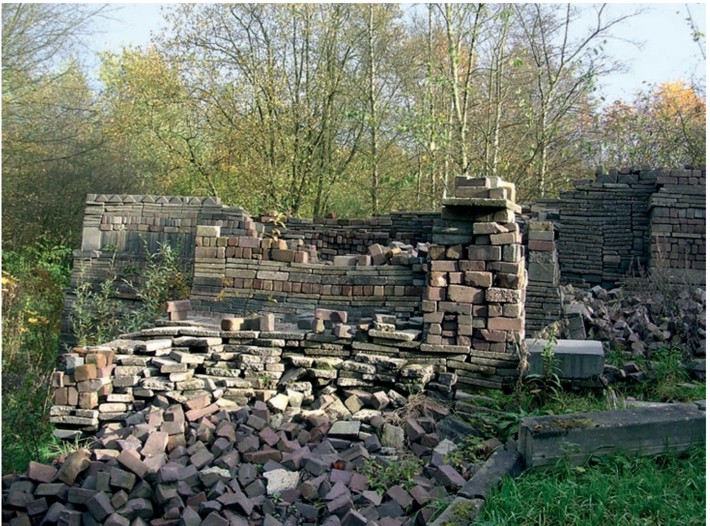
Figure 10: Since the year 2000 there has been considerable progress in building the foundations for the Eco-cathedral. During the summer of that year a large platform or terrace was created by a reunion of Frisian in an open area.
